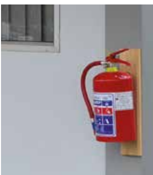
Safety - Fire Extinguishers
